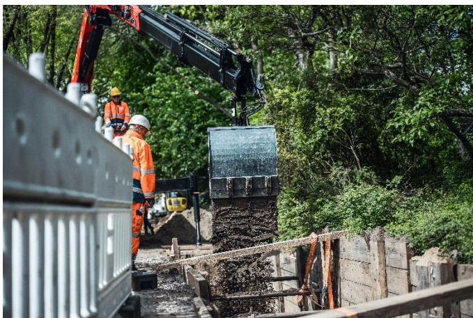
(3) During a pipeline installation project on the Jahnring in Hamburg, the treated soil is reinstalled.
