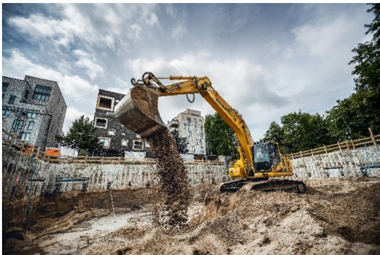
(2) The Bauer Umwelt Division constructed the excavation pit up to a depth of 8 m.
